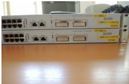
SWITCH SS3 4228G 24port+2 DI1542, DI1543
